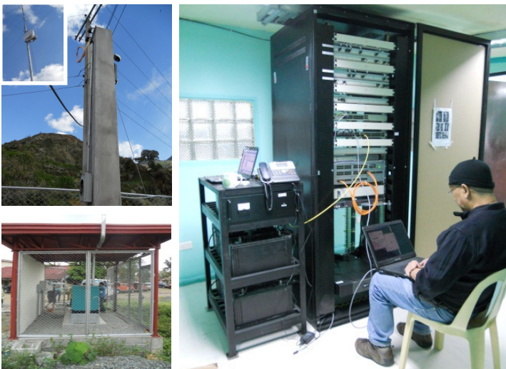
Left (Top): WAN connectivity radio antenna and utility service entrance pedestal. Bottom: Generator power house at the Kalinga District Engineering Office. Right: Network room at the Benguet 2nd District Engineering Office.
