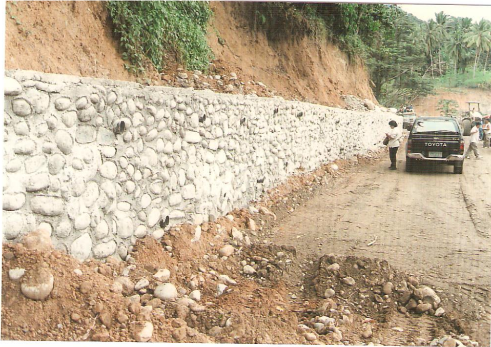
Cobaet Bridge-Gonogon Section last visited by monitors in November 2008. Road is still under construction.
