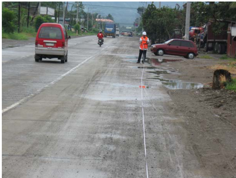
On-going construction in Davao del Norte (Widening/Rehabilitation of Surigao-Davao Road, Apokon Section)
