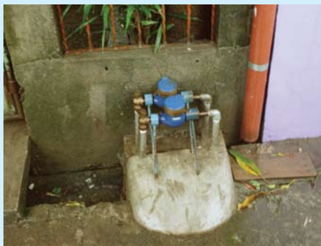
A house water supply connection in Manila.
