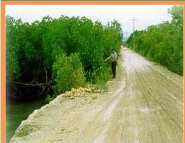
The people of Pangangan Island off Calape, Bohol, have found in mangroves a natural way to protect their island's only road link to the mainland from typhoon damage. The four kilometer long causeway is protected by mangroves planted in recent decades by local schoolchildren.
