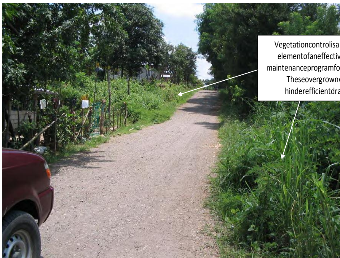
FMR with sideditches covered with overgrown vegetation. (ARCDP2)
