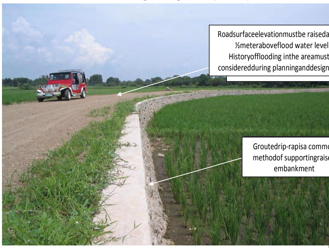
FMR with raised embankments supported by concrete stone masonry or grouted drip-rap retaining walls. (ARCDP2)
