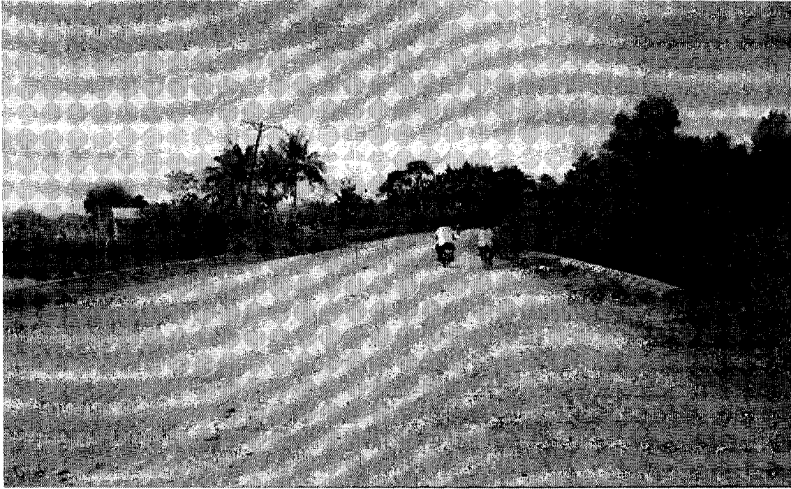
Flood Prone Section to be Upgrade Km. 147 + 050
