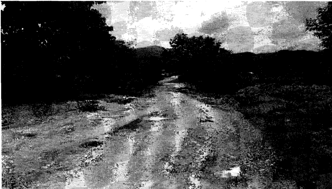
Present Road Condition @ Km. 178 + 000. Brgy. Cabalwa
