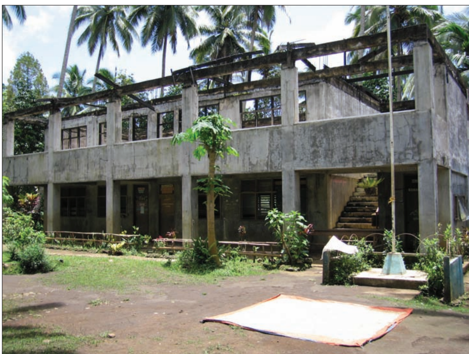
Destruction of a school building. Maguindanao.
