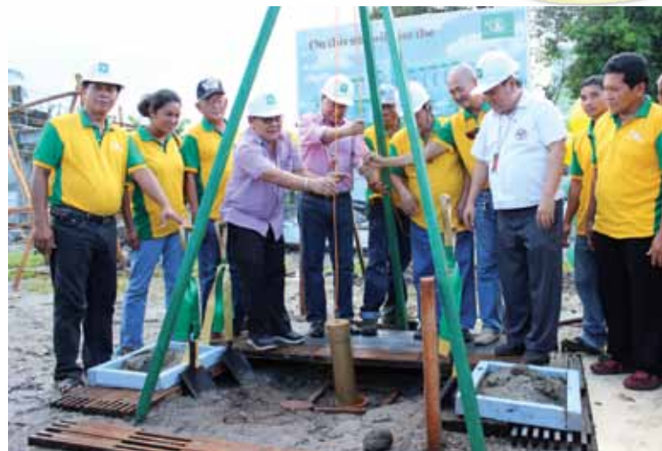
NIA and IA officials in the Bicol region lower the time capsule of the farmers training center during the groundbreaking activity of the edifice.
